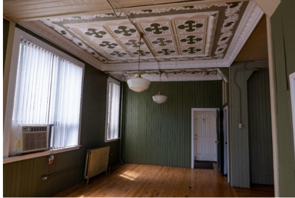
Figure 12: View of wood strip paneling on walls and tin ceilings in the office.
