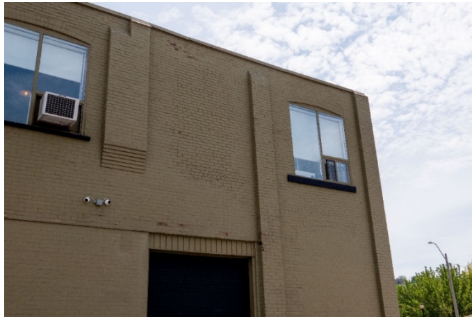
Figure 7: Infilled former window openings at the south end of the west elevation, on both stories.
