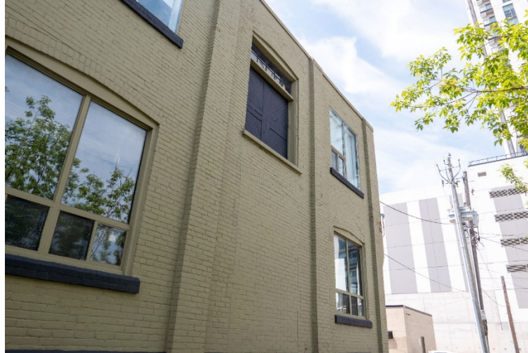
Figure 49: Former openings taller than windows at grade, and the remnant door above suggest loading functions related to the elevator .
